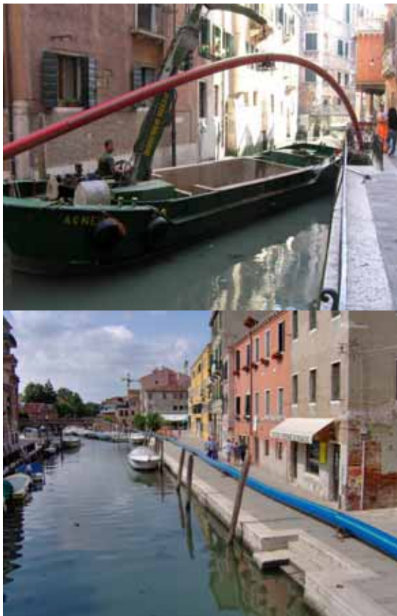
The red fire fighting pipeline (top) and (bottom) the new drinking water supply pipe both provided by egeplast.
