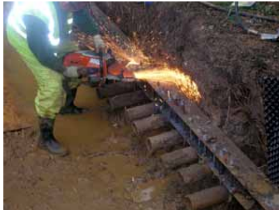
Stabilising of the rootball was achieved by linking the rammed steel pipes together using the RSJ.
