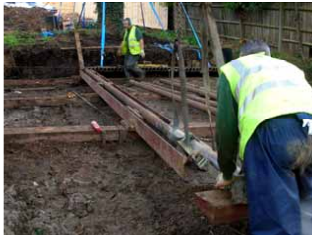
Alignment of the steel pipes was achieved using the guide channel RSJ section in the prepared launch trench.
