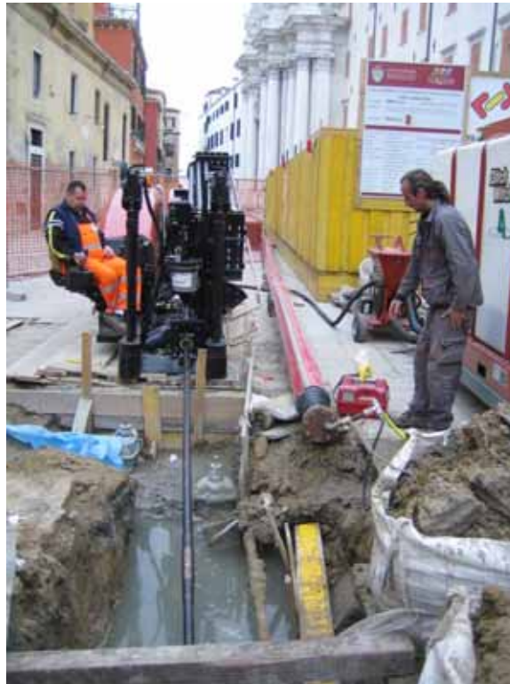
The small start pits used with HDD installation reduced significantly the amount of road excavation required for the project.
