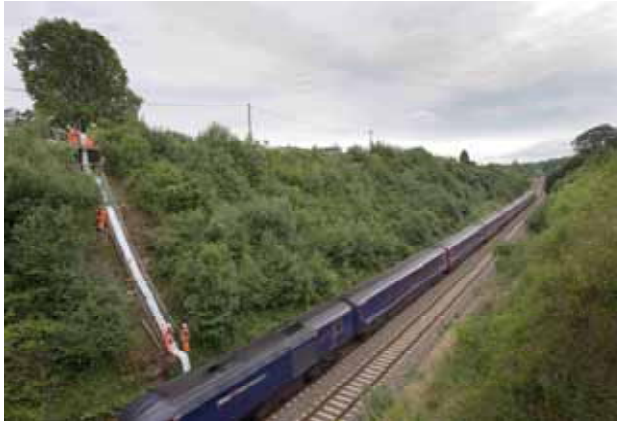
Installing a CIPP lining alongside the active Bristol to London railway line.
