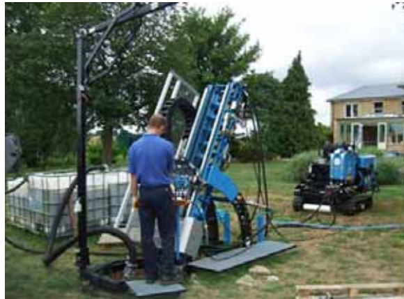
The Geodrill 4R rig positioned on the drilling chamber with Power Unit.
