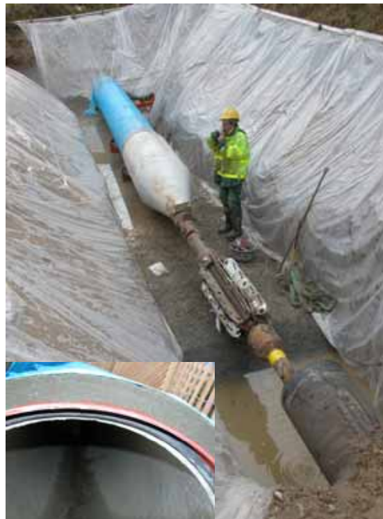
Ready for bursting, the pipe length with the 810 mm diameter expander and the 600 mm diameter cutting blades. Inset a section of the new concrete pipe with steel core.
