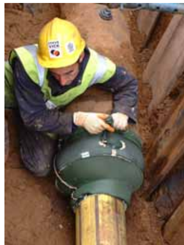
An End Seal being fitted by a Steve Vick International contracting technician.
