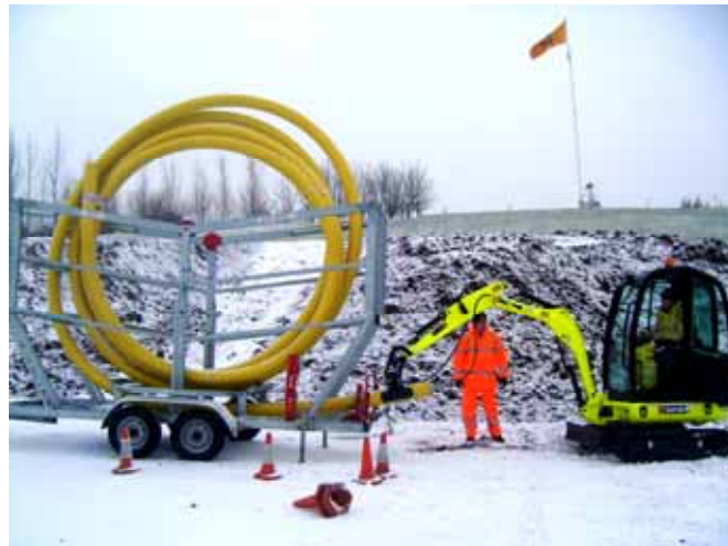
Demonstrating the unloading of a CHUTE ROLLER V-Series Pipe Coil Trailer using JCB equipment.
